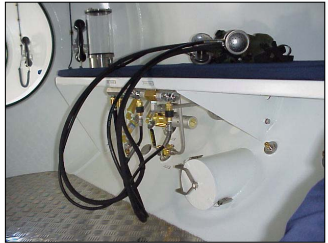
Piping & valves located under bench – main lock
